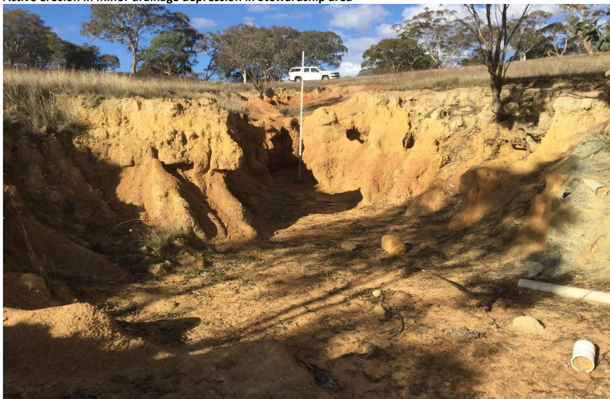
Active gully erosion upslope of Sutton Road in Stewardship area
